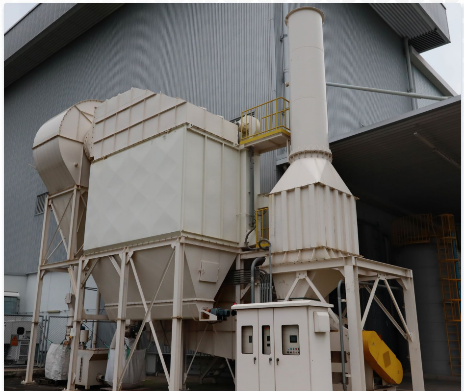
Air Emission Mitigation: Mitigation measures like baghouses help to capture dust particulates generated during the material crushing process.
